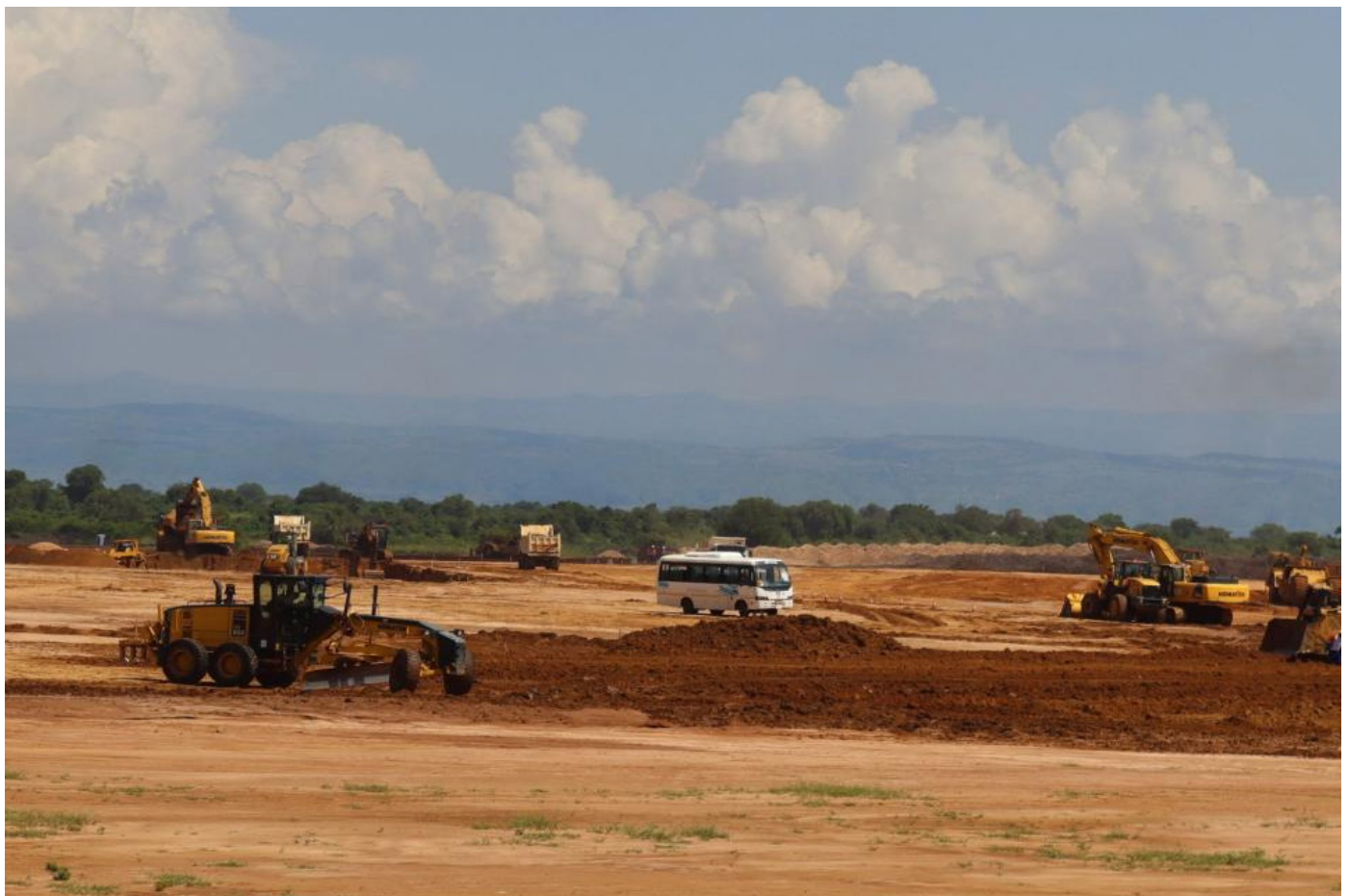
The oil Central Processing Facility (CPF) plant constructed on Uduku 2 and Kasenyi villages –Gwedo community land that displaced more than 640 community residents from 5 villages –Buliisa District".
